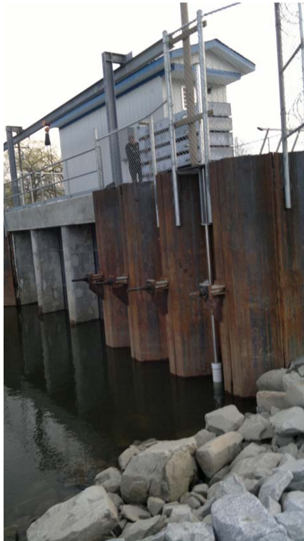
Pump house intake showing Dewidag bars and float level gauge
