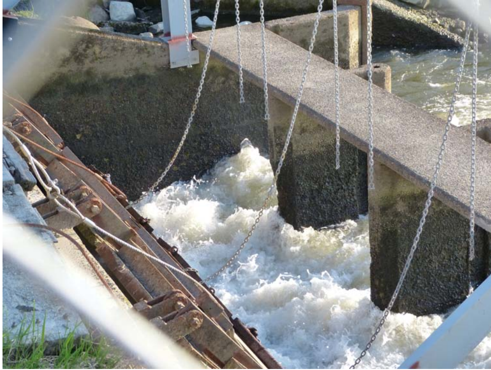
One-way flood gates draining Hatzic Lake into the Fraser River
