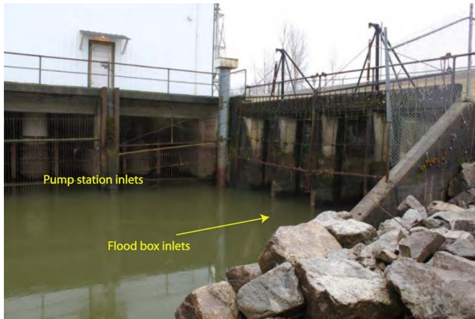
Flood box inlets facing Hatzic Lake. Adjacent to the flood boxes is the Hatzic Pump Station.
