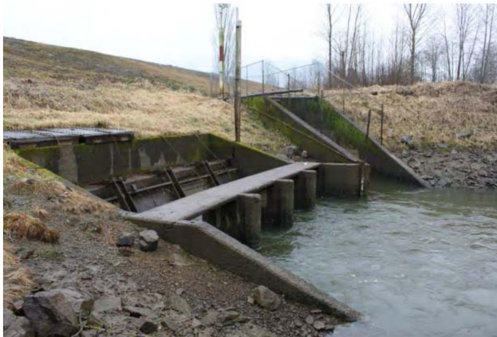
Flood box outlet (Fraser River side), a top hinged flap gate is fitted to the exit of each culvert
